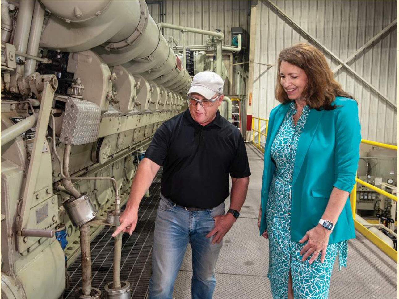
Paul Brunfelt, director of generation for Keys Energy Services, and Tejada tour Stock Island Generating Facility. The site is essential for reliable generation for Key West and FMPA.
